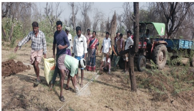
Community members and SEDS staff mark out the tank boundary before excavation begins.
