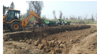
An excavator deepens the reservoir, restoring around 8.7 million litres of water-storage capacity.
