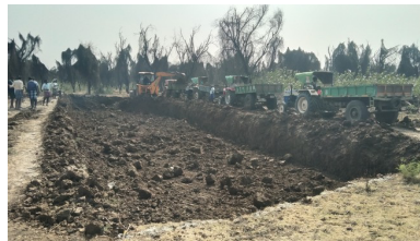
Tractors line up to collect freshly-excavated silt, to be spread as fertiliser on local farmland.
